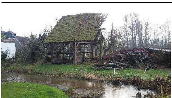
De droogloods is verder ingestort
